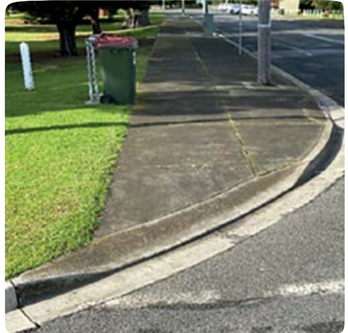
Non-compliant kerb ramp
